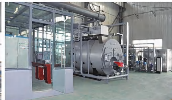
△热工测试平台 Thermal Engineering Testing Platform
