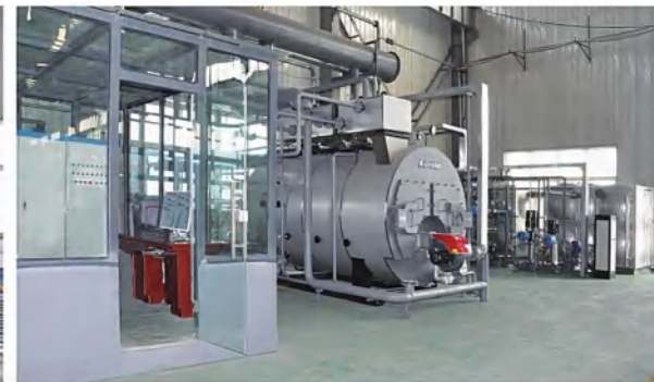
△热工测试平台 Thermal Engineering Testing Platform
