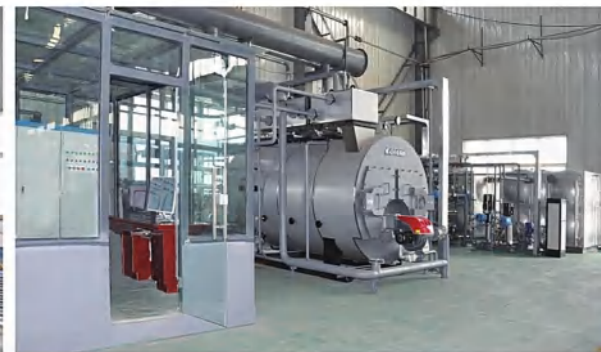
△热工测试平台 Thermal Engineering Testing Platform
