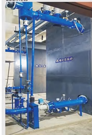
电极锅炉 Electrode Boilers
