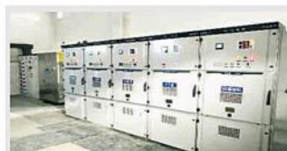
高低压配电柜 High and Low Voltage Distribution Cabinets
