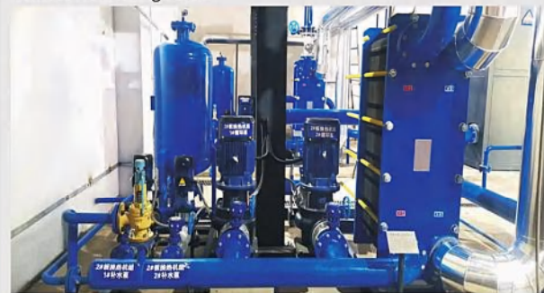
换热机组 Heat Exchange Unit
