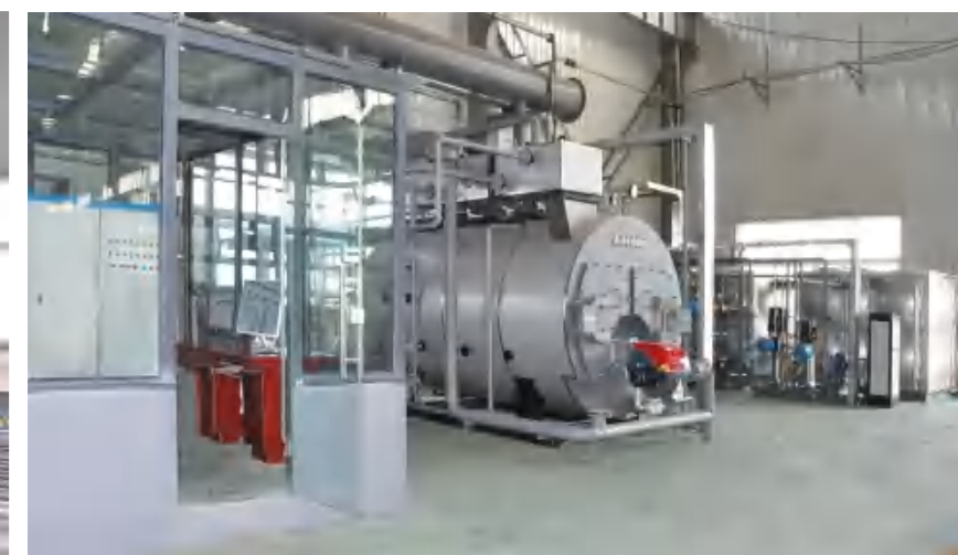
△热工测试平台 Thermal Engineering Testing Platform
