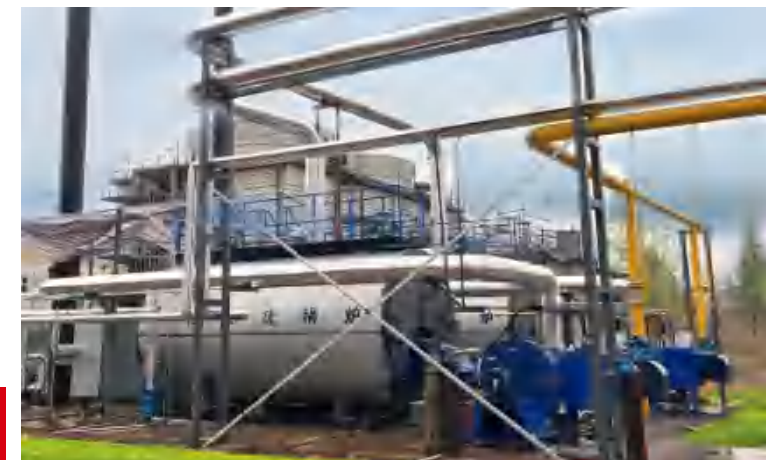
燃纯氢气锅炉现场 On-site Photo of Pure Hydrogen-Fired Boilers
