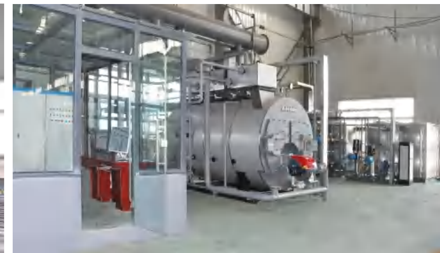
△热工测试平台 Thermal Engineering Testing Platform
