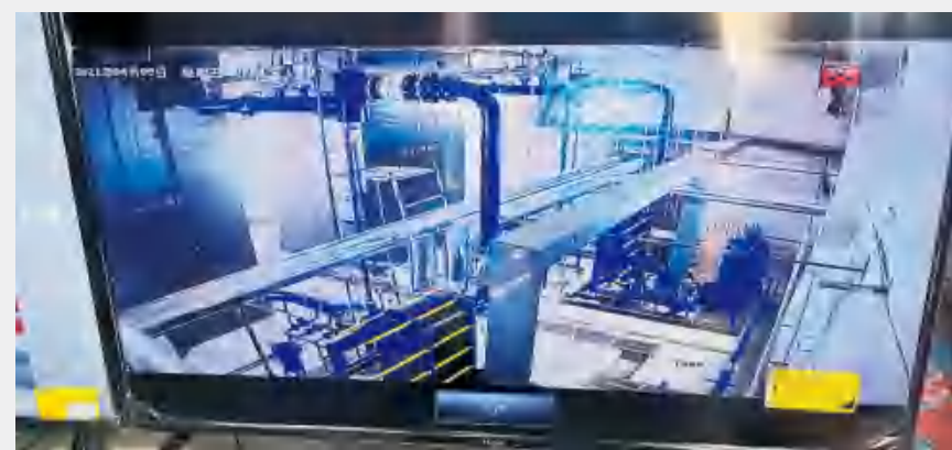
远程监控画面 Remote Monitoring Screen
