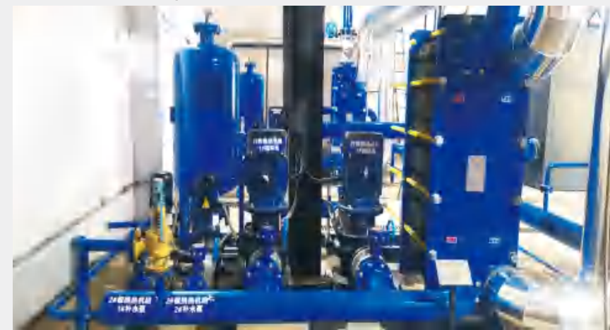
换热机组 Heat Exchange Unit
