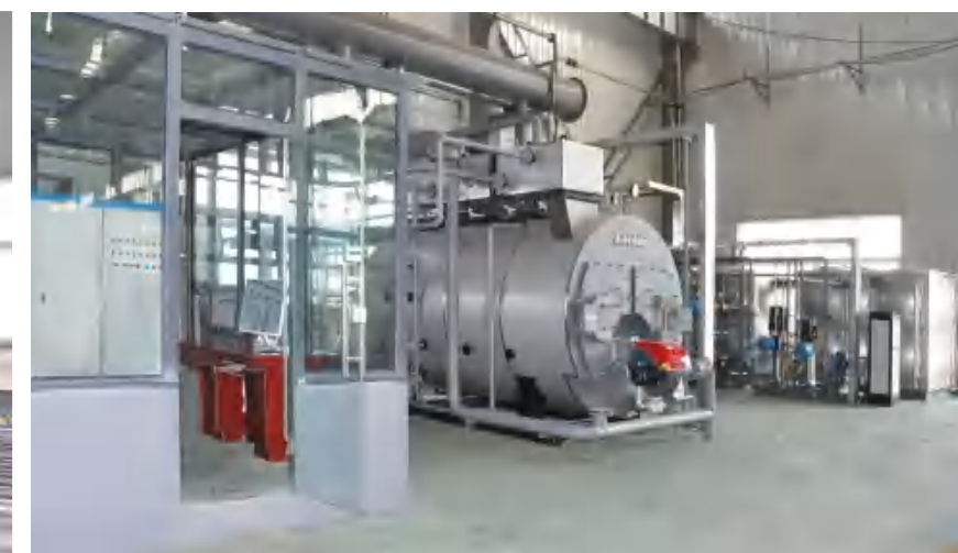
△热工测试平台 Thermal Engineering Testing Platform
